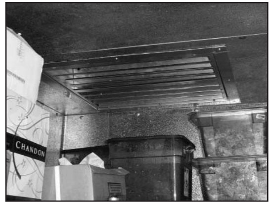
Inside view of an installed walk-in cooler.
